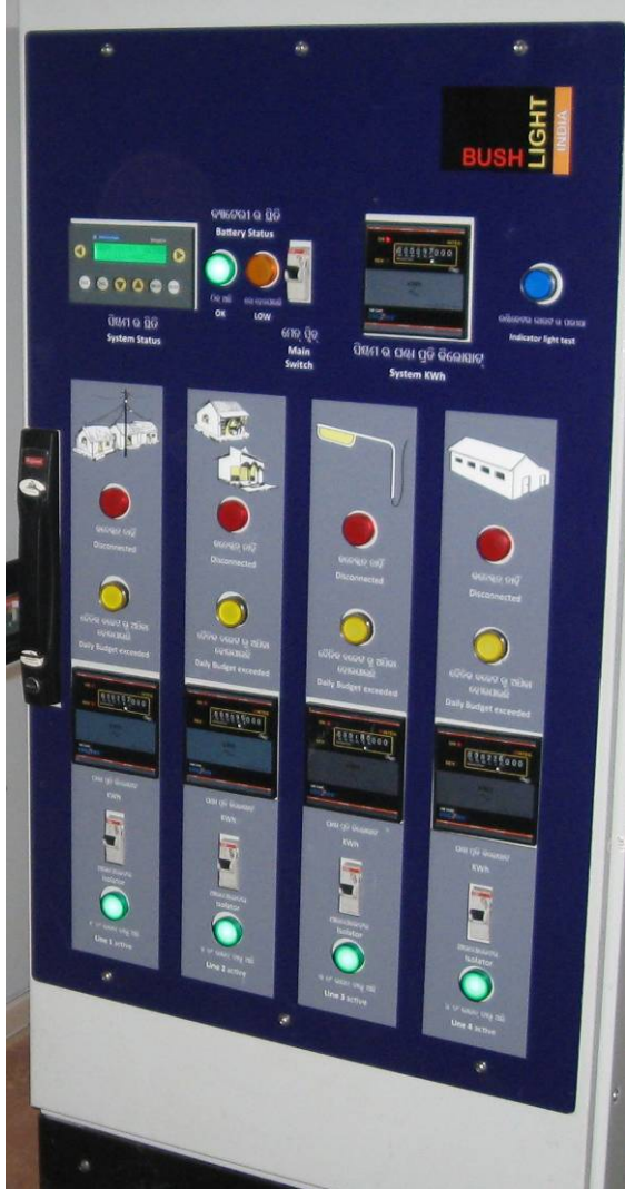
Figure 6: The System Control Board – centralised control and distribution board.
