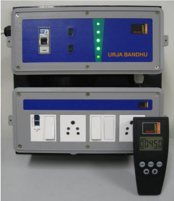
Figure 5: The Urja Bandhu energy meter with integrated switchboard and universal UB Programmer.
